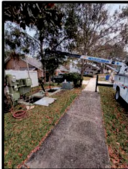
Removed Rags from LS #30 Pumps #1 & #2
