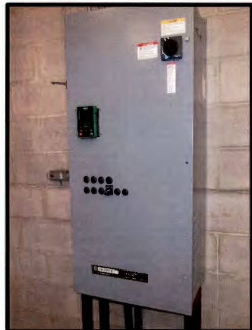
New Curlew Reuse pump VFD's installed
