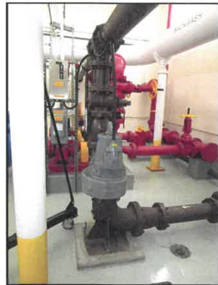
New Mudwell Pump #1 Installed at Fac #16 Dirty Backwash Basin
