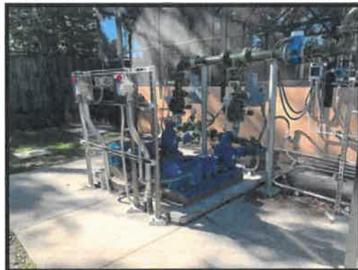
New Media Decant Pump System
