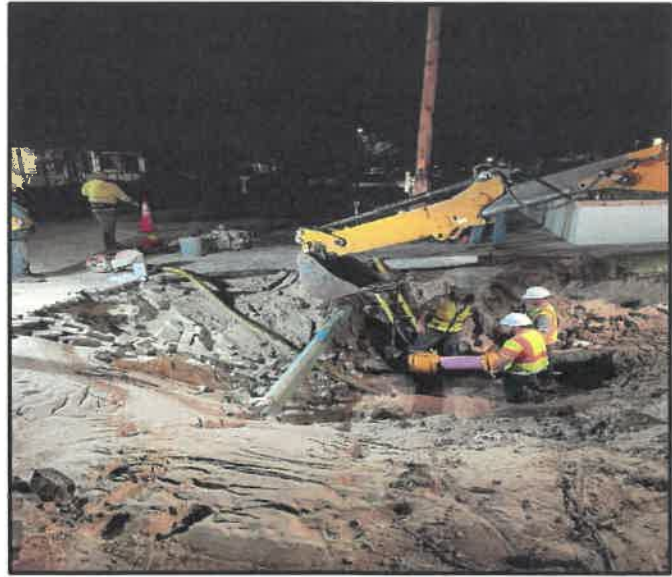
Reclaimed Water Main Break 654 Scotland Street
