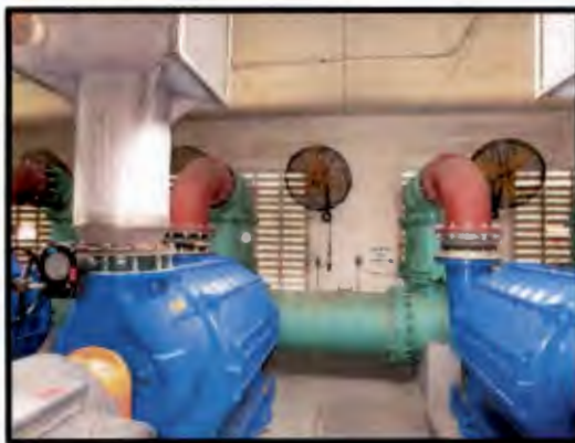
Fac 13 Blower Building Fans x5 Installed for Circulation
