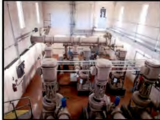
Fac #7 Sludge Building Fans x3 Installed for air Circulation
