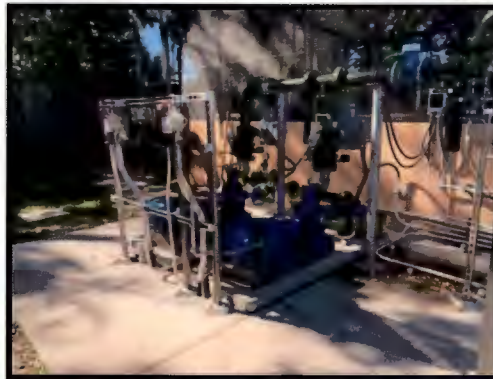
New Media Decant Pump System
