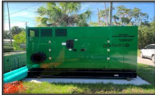
Pictured above - City of Dunedin , Lift Station #8 Standby Emergency Pump
