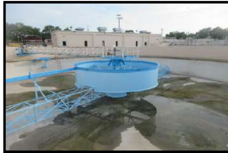
Wastewater Treatment Plant- North Clarifier
