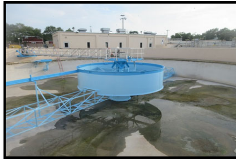
Wastewater Treatment Plant- North Clarifier
