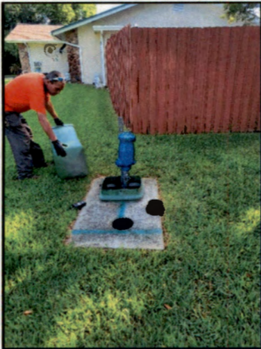
ARV Repair #3 Beltrees Street
