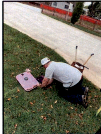
Reclaimed / Backflow Inspection 1196 Robmar Road
