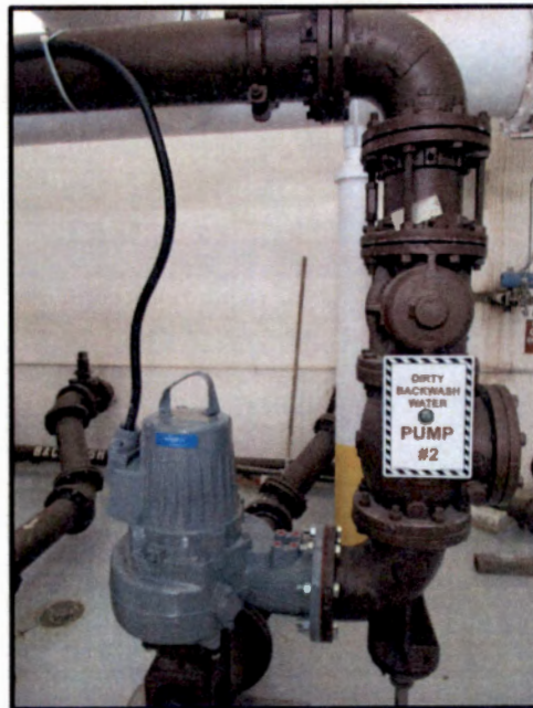
New Flygt Pump #2 Facility #8 Filter Building
