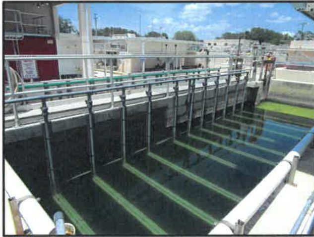
New South Reaeration Tank Air Header System Installed Fac #10
