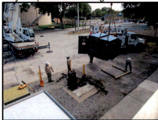
New Duke Energy 2500 KVA Transformer Installed
