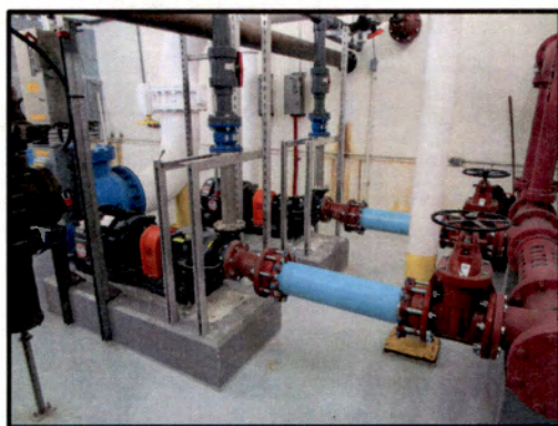
New Reuse Isolation Pumps Facility #8 (Filter Building)
