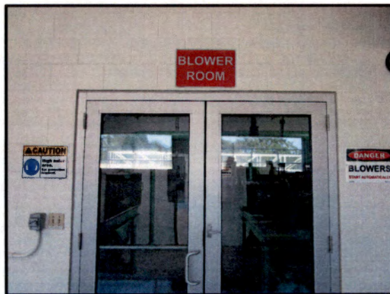
New Safety Signs at Facility #8 Blower Room
