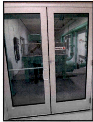
New Hurricane Impact Doors Facility
