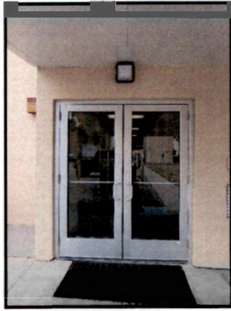
New Hurricane Impact Doors Facility #2
